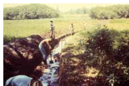
(Figure 5) Reconstructing a drainage canal in order to provide a permanent waterway promoting the free-flow of water through a malaria-prone region. Source: CDC (1981)
